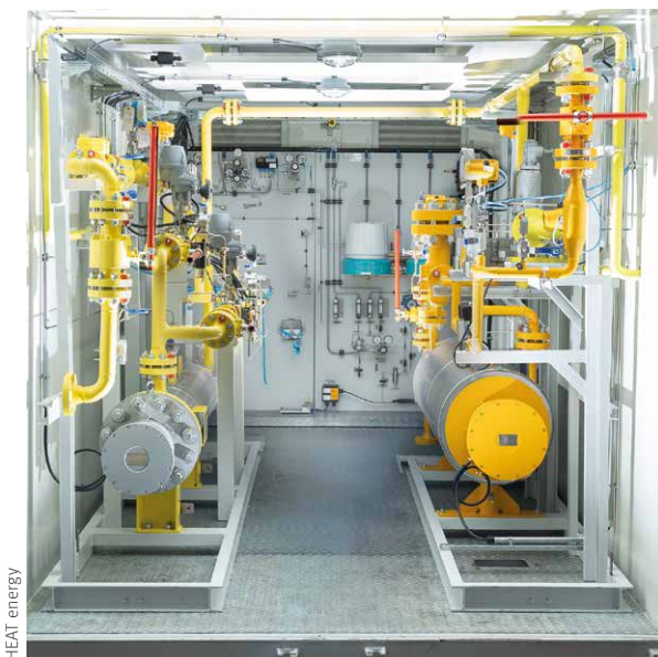
Abb. 2 Biomethan Container- station HEAT energy
